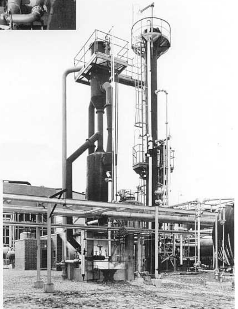
A two-stage self-supporting CHILL-VACTOR is installed in a paper-mill chlorine dioxide bleaching process.
