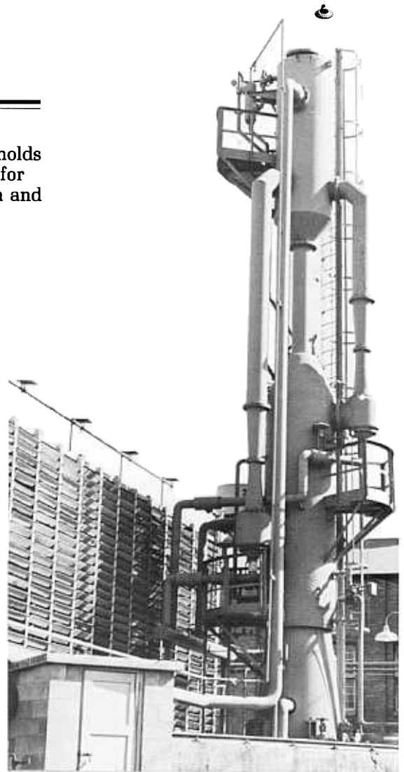
200 ton C-R CHILL VACTOR steam jet refrigeration unit chills water for bleaching operations at Crown-Zellerbach Corp.
